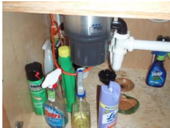
The disposer is not wired safely
