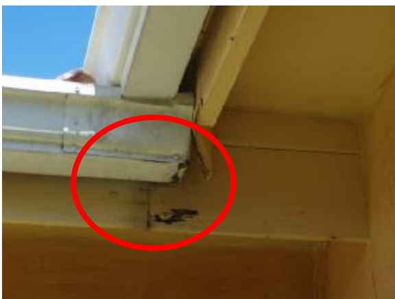
The water damaged wood.
