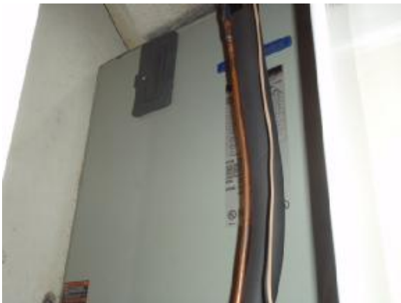
View of the air handler
