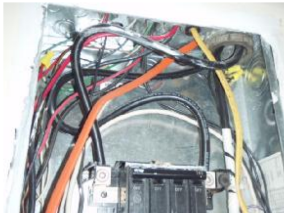
Splices in the panel need correcting.
