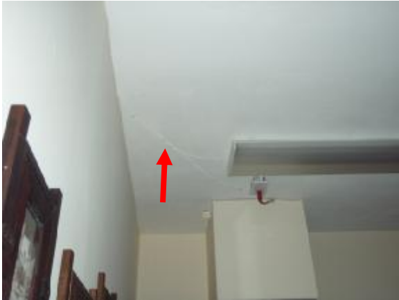
The Romex wire is installed improperly
