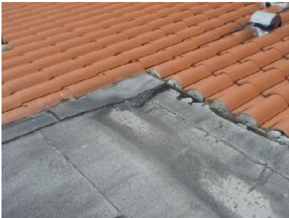
The flat roof is deteriorated.
