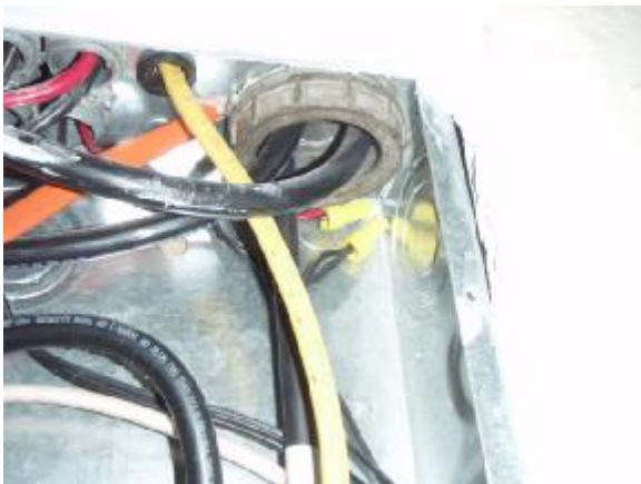
The Romex wires are improper in the panel.
