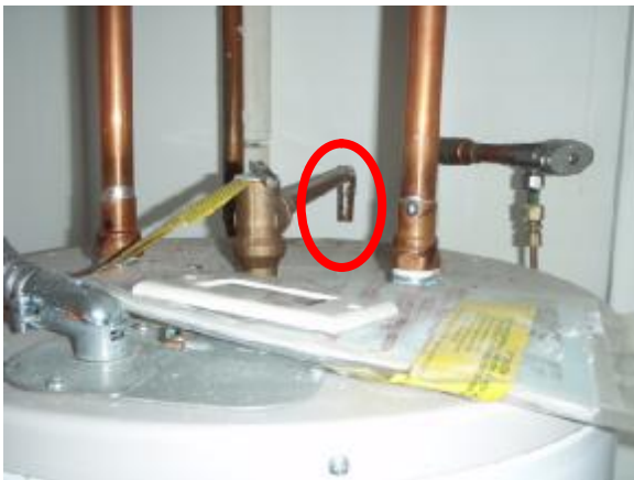
The TPR pipe requires repair
