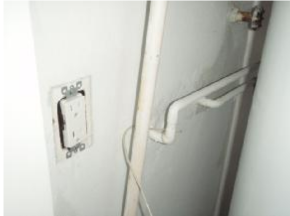
Replace outlet covers
