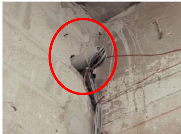
The conduit penetration requires fire stop caulking.
