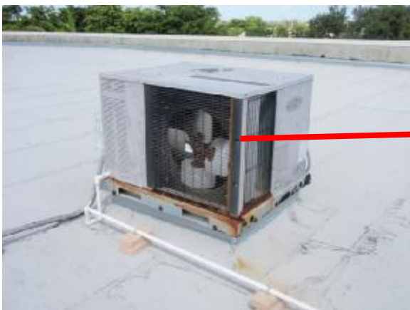
View of the older a/c's
