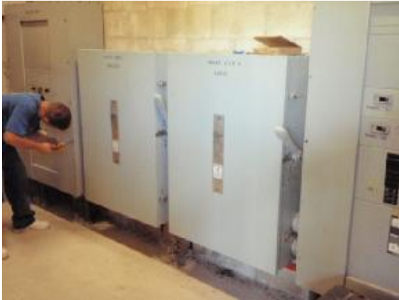
Main panel room
