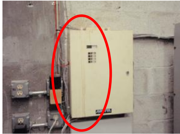
Drip stains from the leak.
