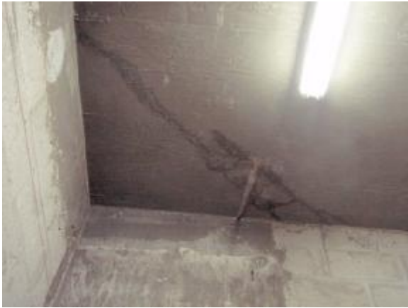
The roof leak at the main panel room.
