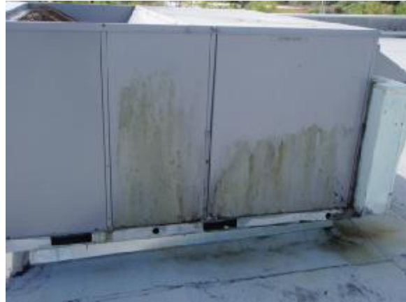
Signs of previous leaks.
