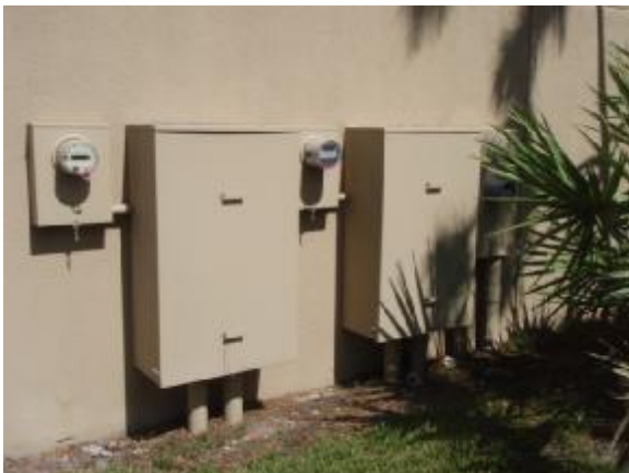
The exterior meters
