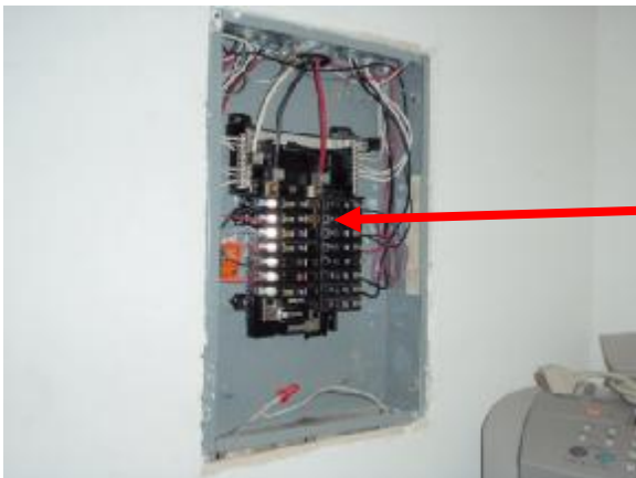
This panel is all overheated and needs replacement.
