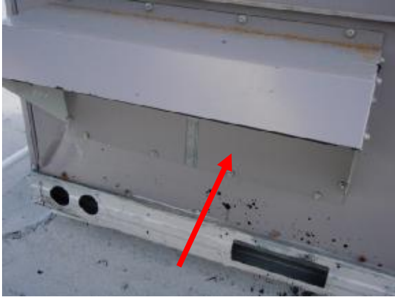
The fresh air intakes should be open.
