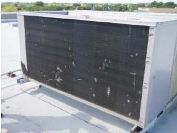
The damaged coils
