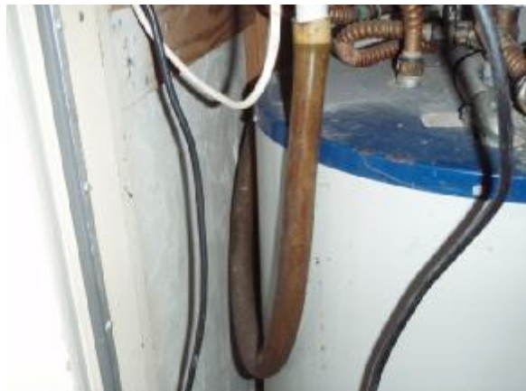
The a/c condensate line is clogged.
