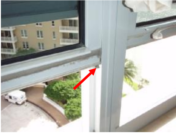
Damaged window spring.
