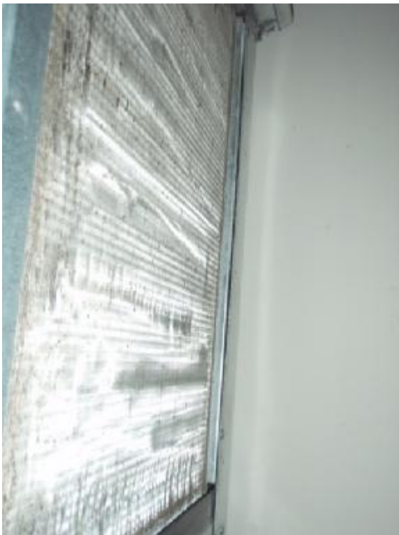
The damaged a/c coil.
