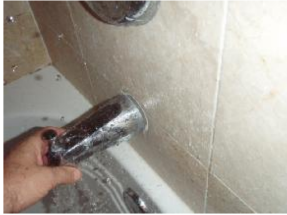
Tub spout loose.
