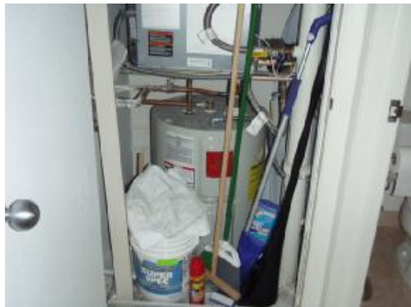
The a/c closet should be clean and not used as storage
